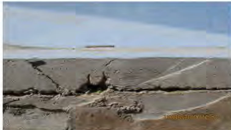
Figure 6: Gap between the distribution channel and precast slab. The cracked triangular wedge leading down from the top of the slab indicates grout used to fill the gap between adjoining precast slab units.
