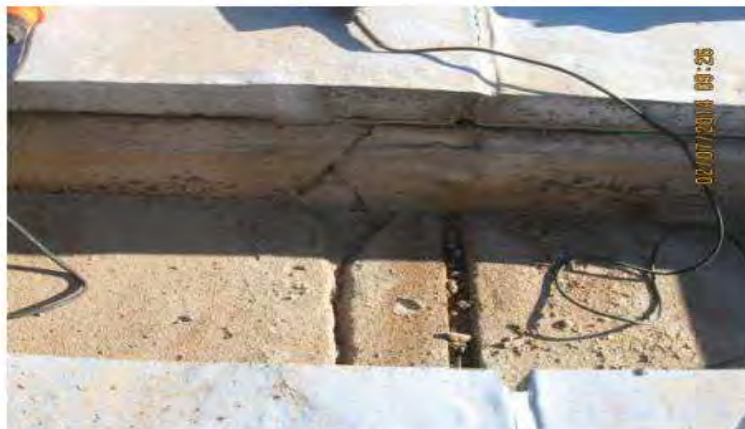
Figure 3: Precast slabs over the distribution channel were locally removed to expose damage to the construction joints.
