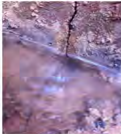
Figure 1: Breach In East construction joint found In May 2014.
