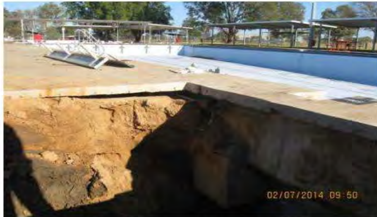
Figure 2: Soil subsidence under the coping slab on the East side near the damaged construction joint.
